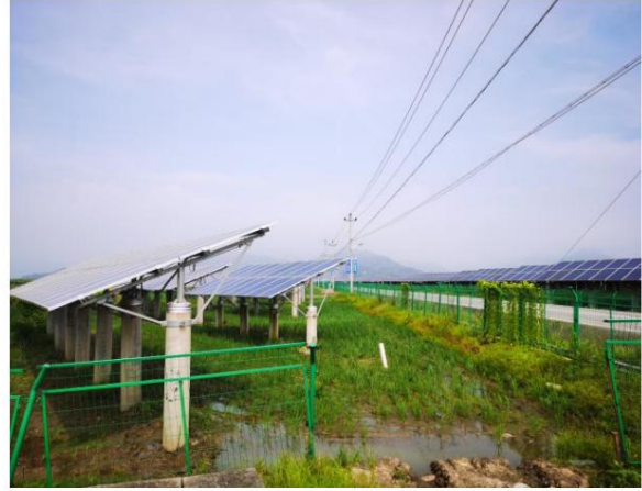
Figure 1-8 Recultivation under photovoltaic panels
