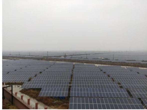
Figure 1-2 Current status of photovoltaic area
